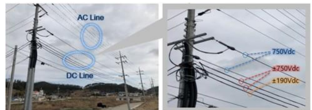
Fig. 5 DC line installation on electric pole
