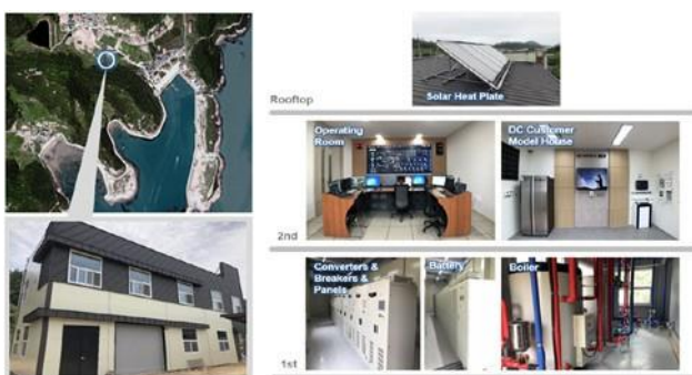
Fig. 9 EV, V2G station and LED street light in DC Island
