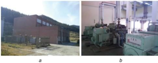
Fig. 1 (a) Existing power plant of the island, (b) Aged three diesel generators
